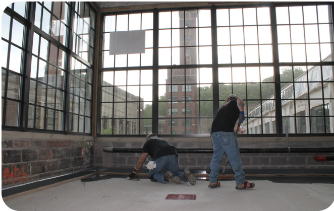
The coating system in the taproom areas again required squeegee and backroll method, this time with two coats of Sherwin-Williams GP 3477 epoxy sealer, each at 3–4 mils (76.2–101.6 microns) DFT.
