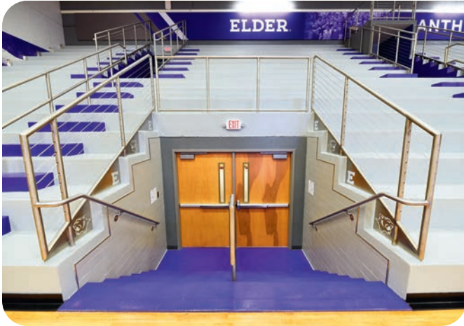
Areas adjacent to the court were coated using a squeegee-and-backroll method instead of spraying. Other trades were onsite, too.
