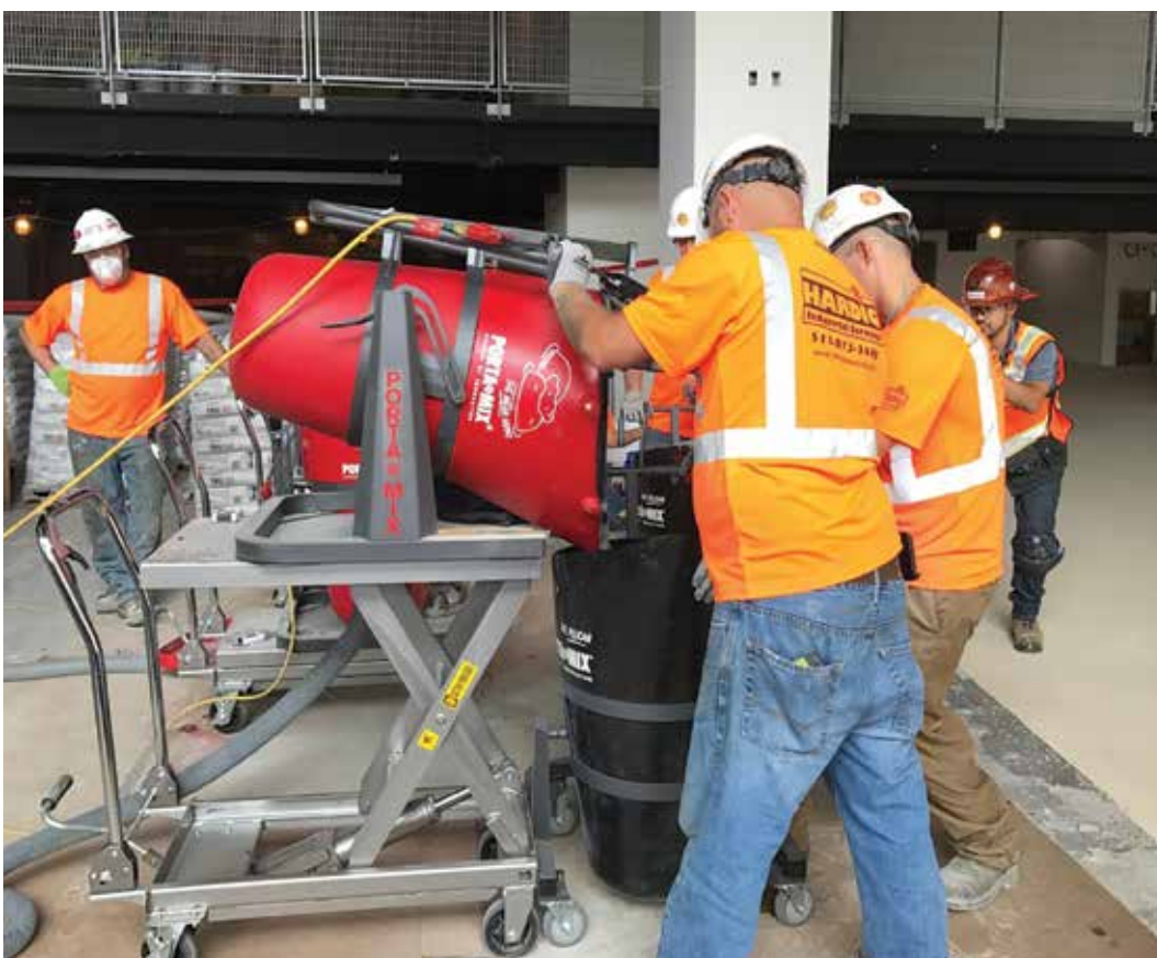
The scope of the project included the installation of Sika Purcem Decoflake UEF, medium finish polished concrete, Rapid Set Tru PC polishable overlay and self-leveling underlayment placed under the permanent basketball court. ALL PHOTOS: HARDIG INDUSTRIAL SERVICES
